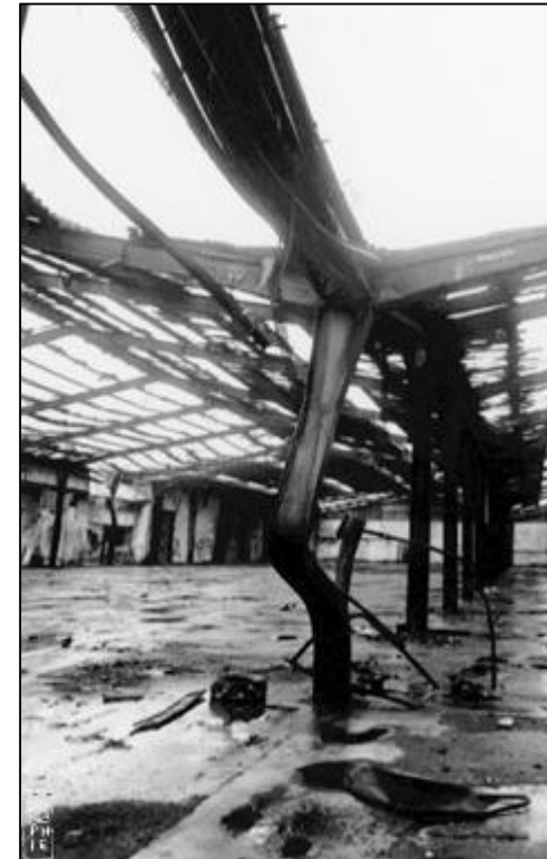
Flambement d'une colonne (Source: Interdisciplinary Research Drivers and Serendipity Factor: An Applied Mechanics Perspective , Chih-Kung Lee & al.)
