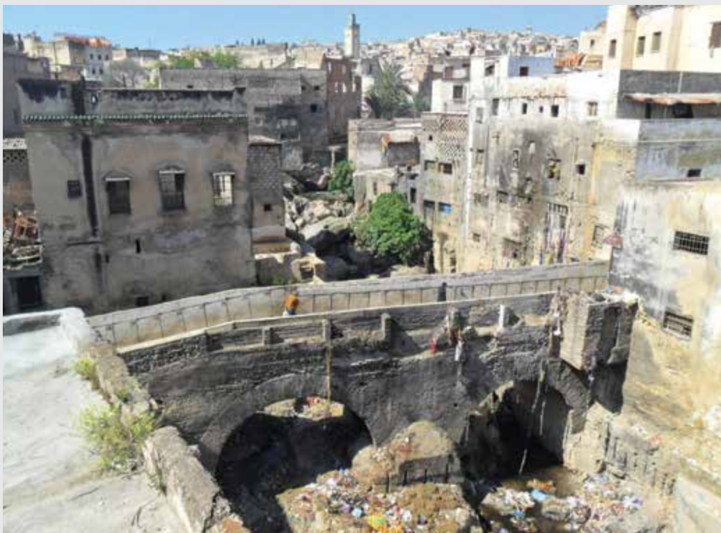
View of Bim Lamdoun Bridge and of Place Lalla Ydouna in Fez Medina
