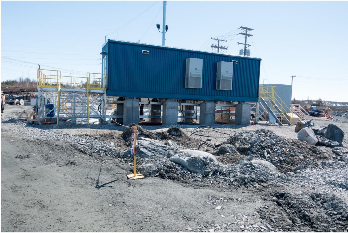
Figure 18.8 – 4.16 kV Switchgear Building
