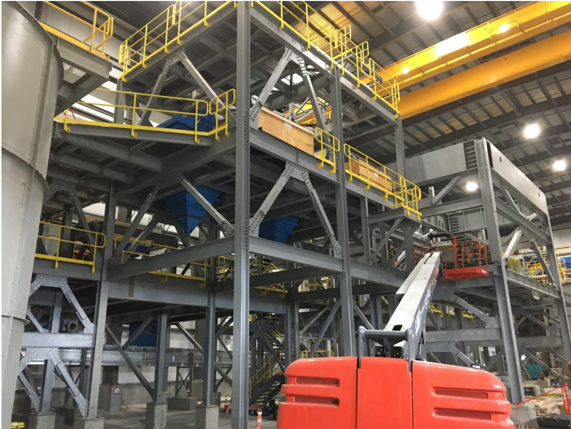
Figure 24.12 – View of the Hydraulic Separators
