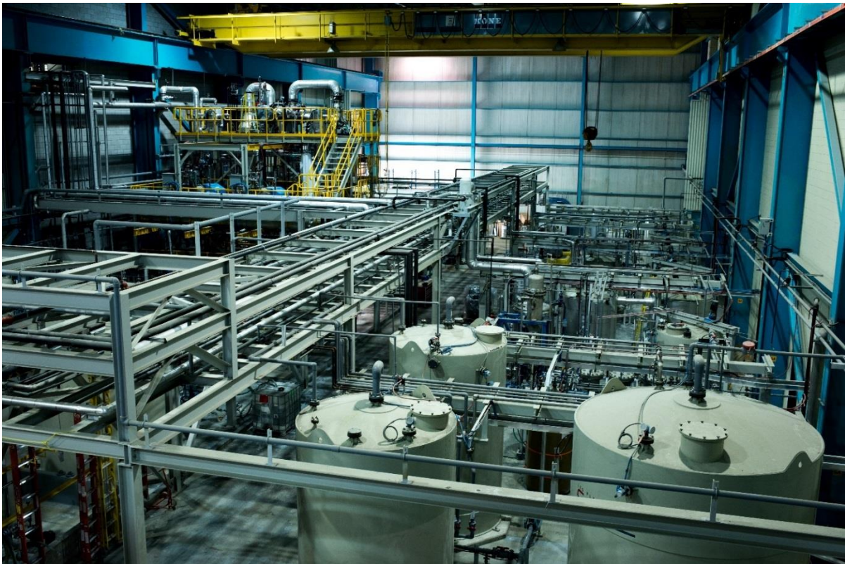
Figure 1.3 – Phase 1 Plant Overview Picture - Purification and Crystallization Unit Operation
