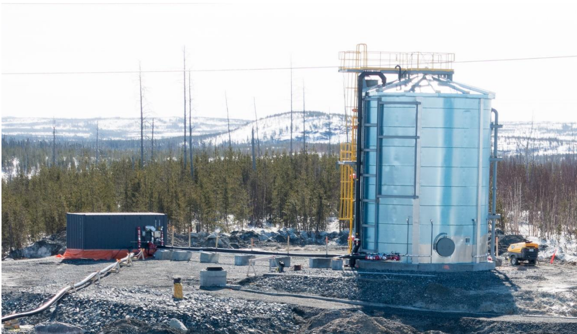
Figure 18.4 – Fire Water / Fresh Water Tank
