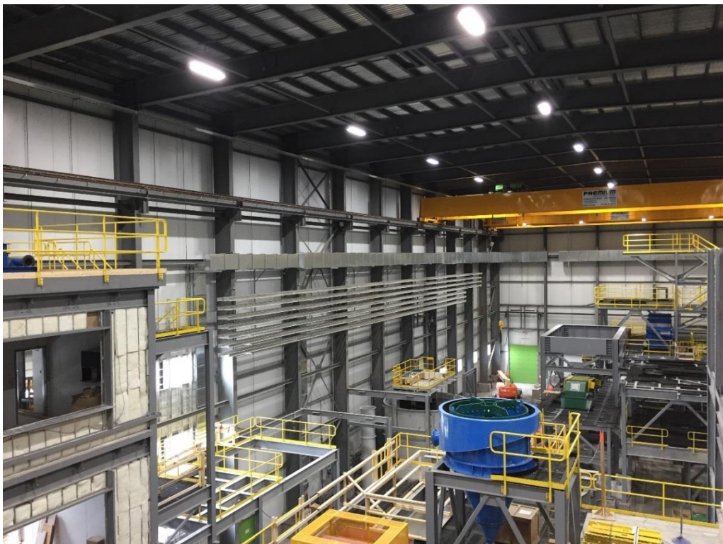
Figure 24.5 – View of Concentrator Interior
