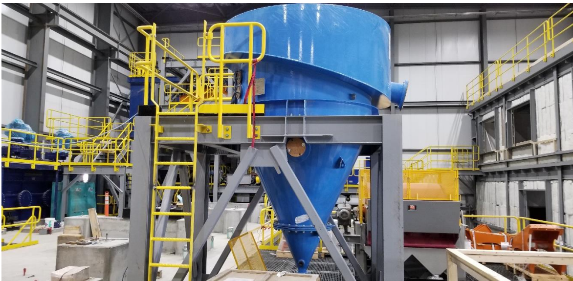
Figure 24.11 – View of the Hydrocyclone
