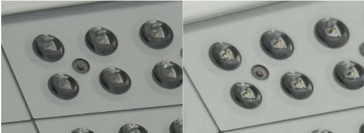
Figure 30. Smart Road LED luminaire before (left) and after (right) cleaning with an IPA rag (Cleaning Method 3), clearly showing removal of gray-colored dirt from the optics.
