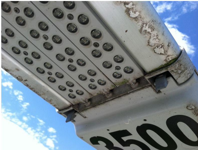
Figure 27. Dirt accumulated on Smart Road LED luminaire type A (3500K).
