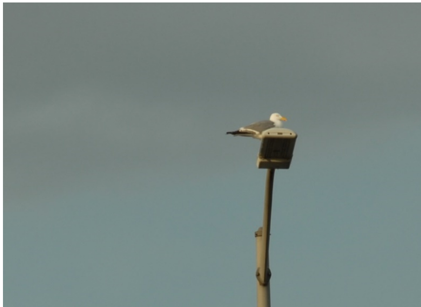
Figure 58. Bird perched on a luminaire heat sink.
